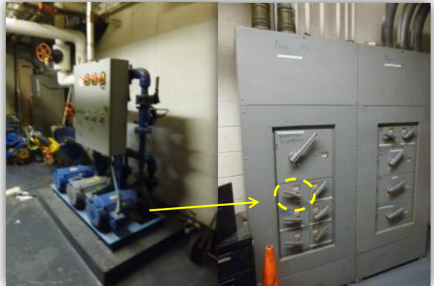
Water Booster Pumps
