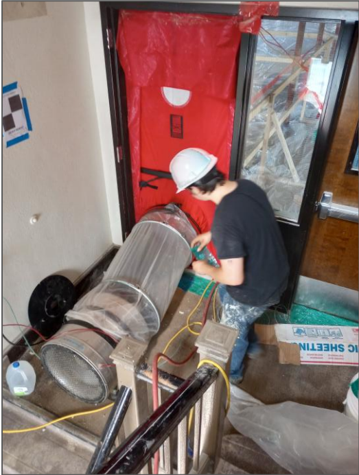
Blower Door & Fan Installed in Stairwell
