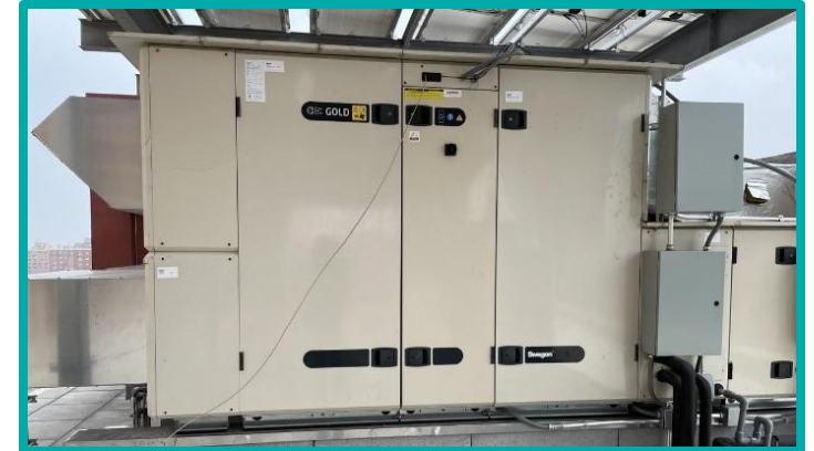
Energy Recovery Ventilator (ERV)
