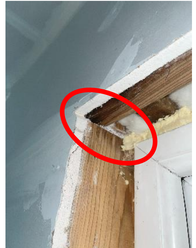
Around exterior door
