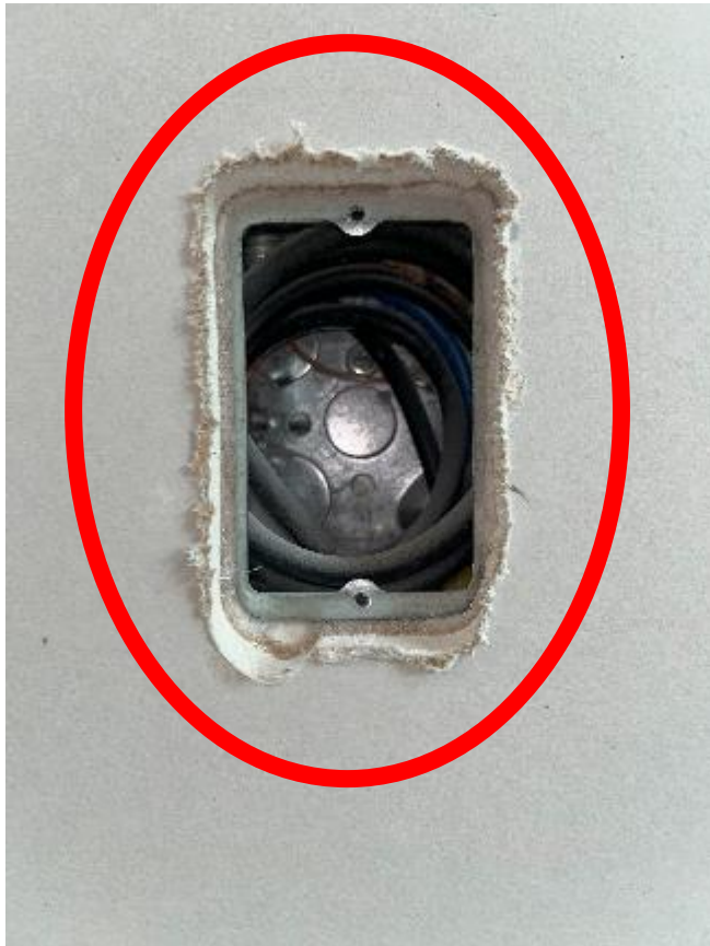
Around electrical box
