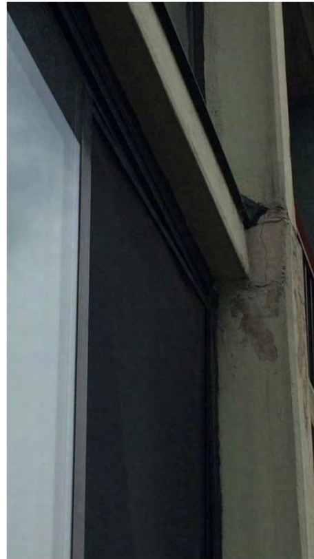
Cracked pre-cast panel
