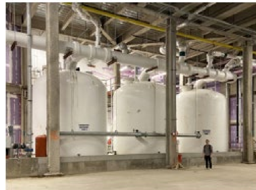
78,000 Gallon Water Collection System
