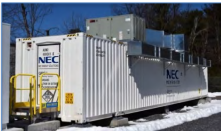
Sterling 2 MW / 3.9MWh ESS Community Resilience Grant
