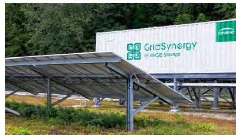
Holyoke 3 MW / 6 MWh ESS Peak Demand Grant
