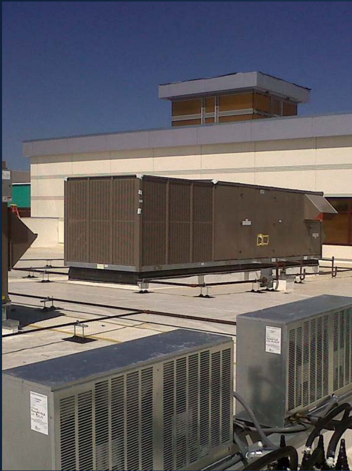
Building Systems Commissioning
