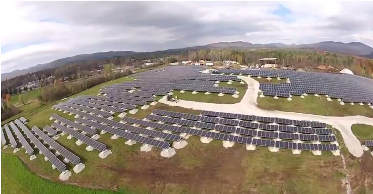
Stafford Hill 2 MW Solar Farm
