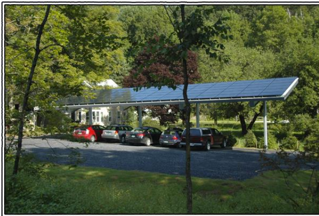
Solar carport & 1 Tracker – 19 kW
