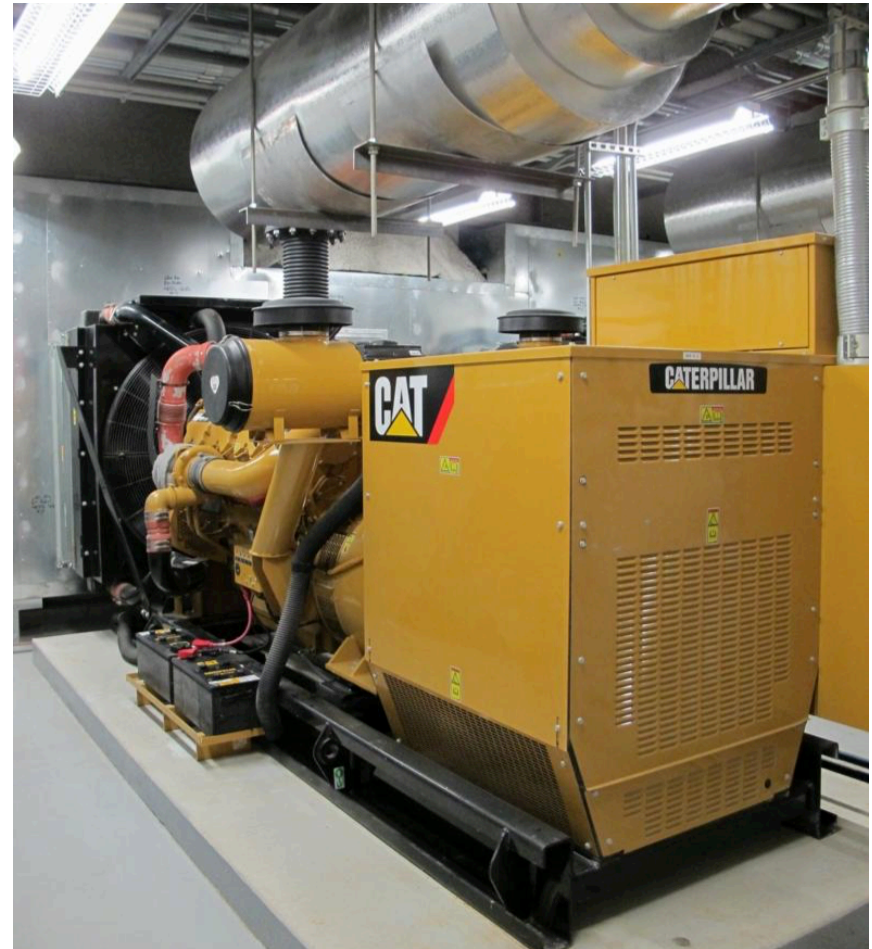
250-kW generator at Spaulding Rehab.
