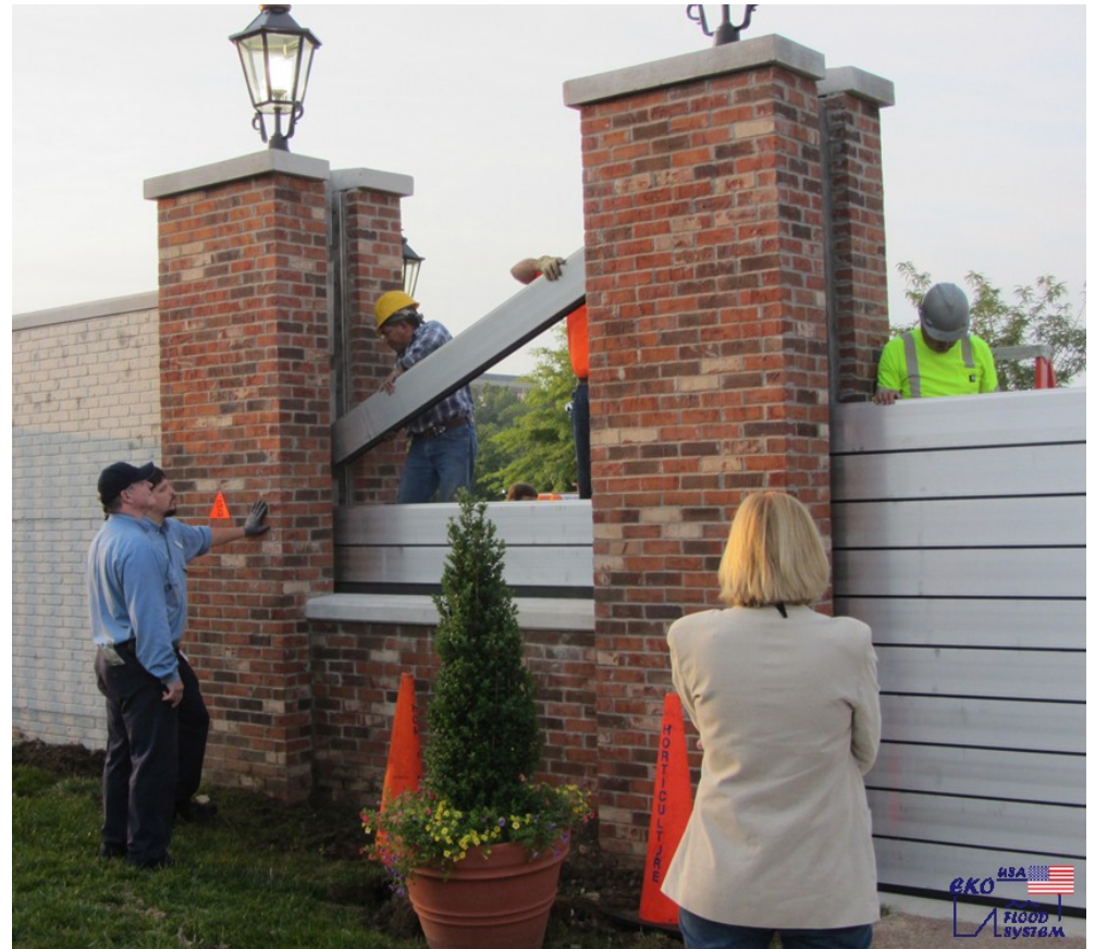
Deployable flood barriers in Nashville - photo: EKO Flood, USA
