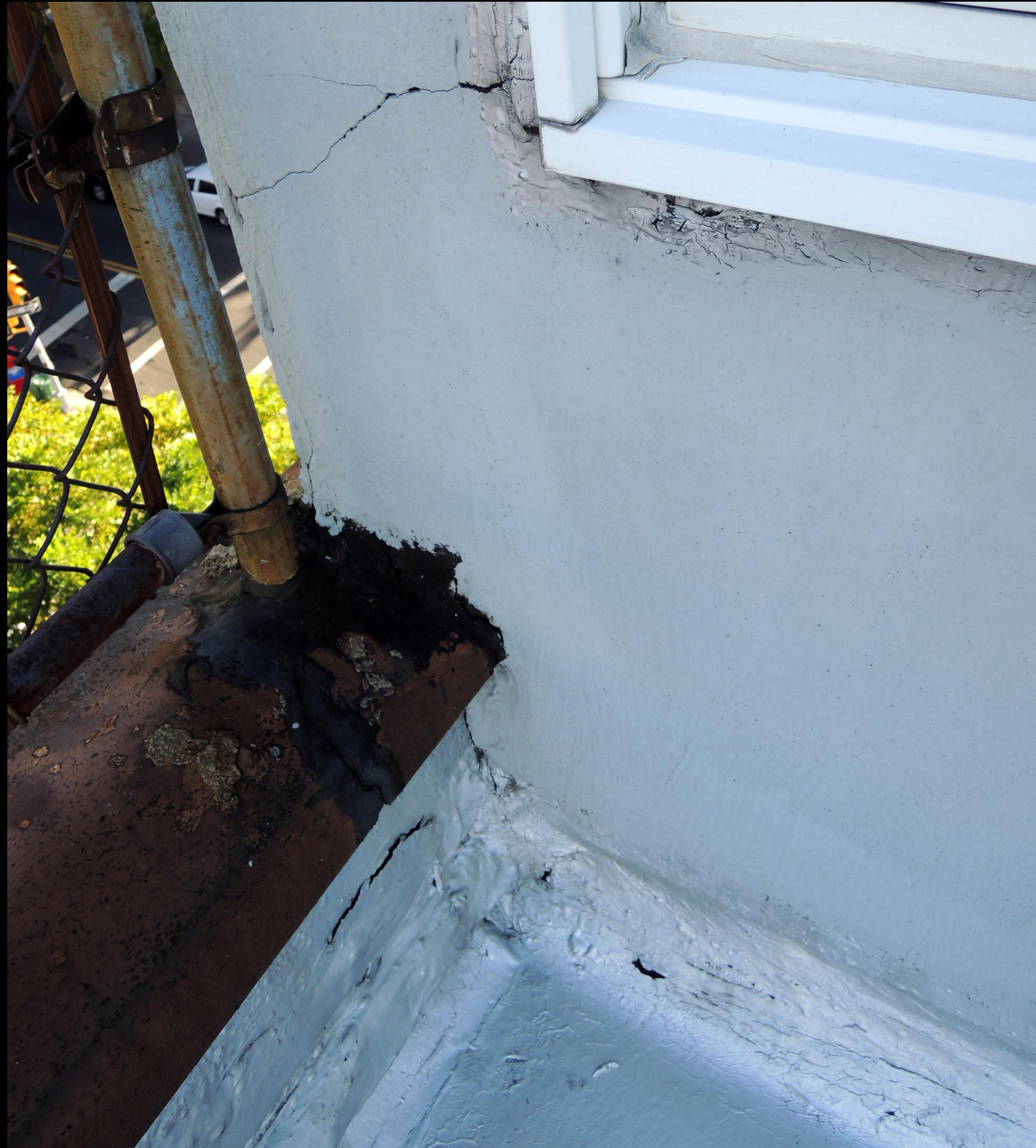
Typical Railing Details. Poor design. Poor execution. Lack of maintenance.
