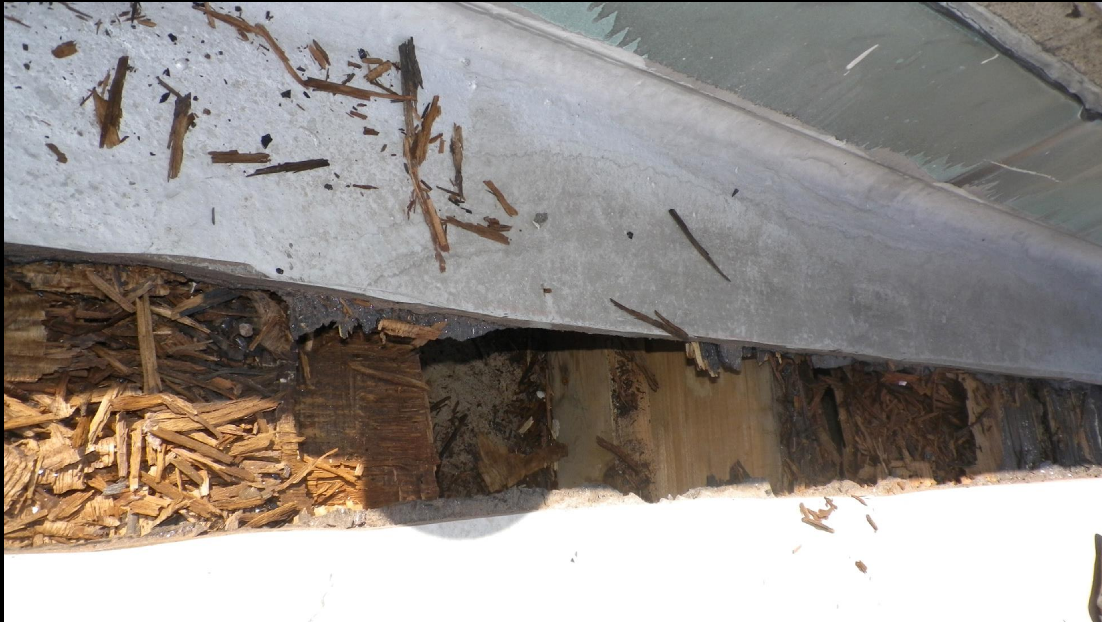
Rotted wood deck due to the improper base flashings. Leaking parapets and unprotected coping stones are to blame.
